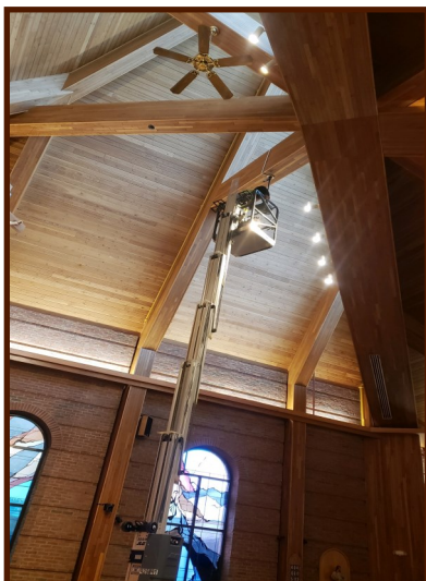
AN ELECTRICIAN RECENTLY INSTALLING A NEW CEILING FAN IN THE UPPER SANCTUARY
